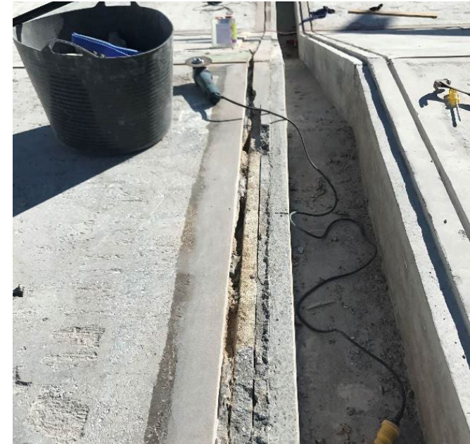
Investigate and report on condition of centre feed line channel. Propose solution to remediate.
