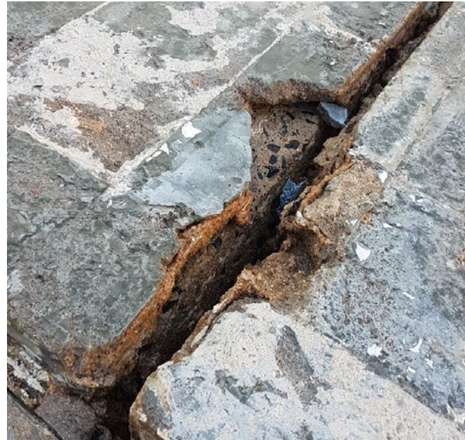
Investigate and report on condition of construction and expansion joints. Propose solution to remediate.
