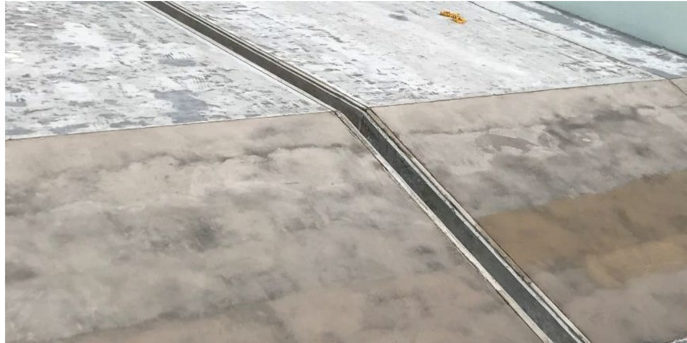
Installation of Epoxy resin system applied to the complete floor surface prior to priming.
