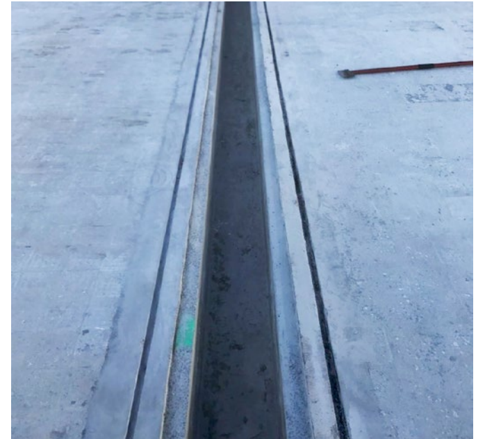
Rebuilding of channel base and walls with Epoxy resin system. Re-cut new joint detail to match original profile.
