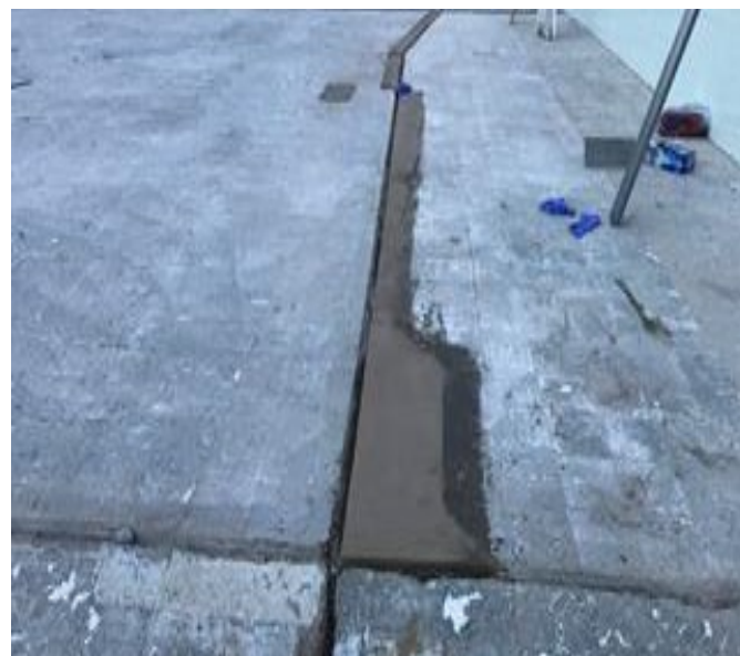
Epoxy Joint Repair - Troweled off to Match Original Substrate and Joint Profile.
